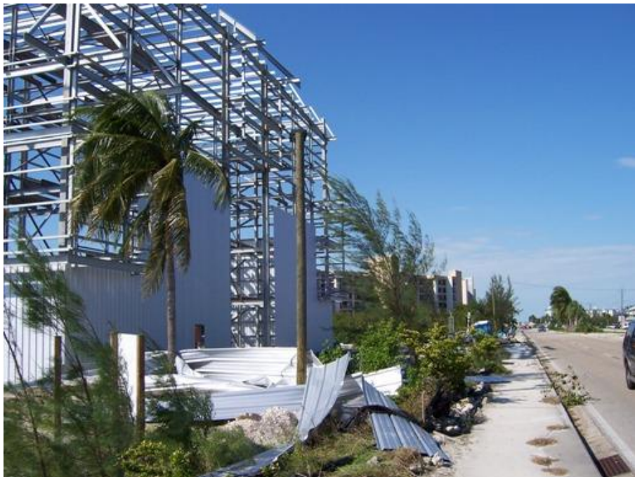
Figure 3. Damage to aluminum sided building in Bonita Beach, FL from Hurricane Wilma.
