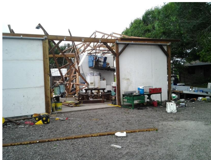
Myakka City tornado damage.
