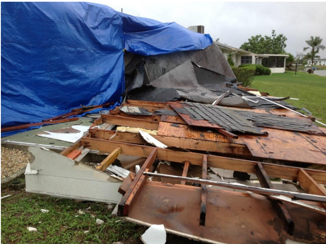
Sun City Center tornado damage.
