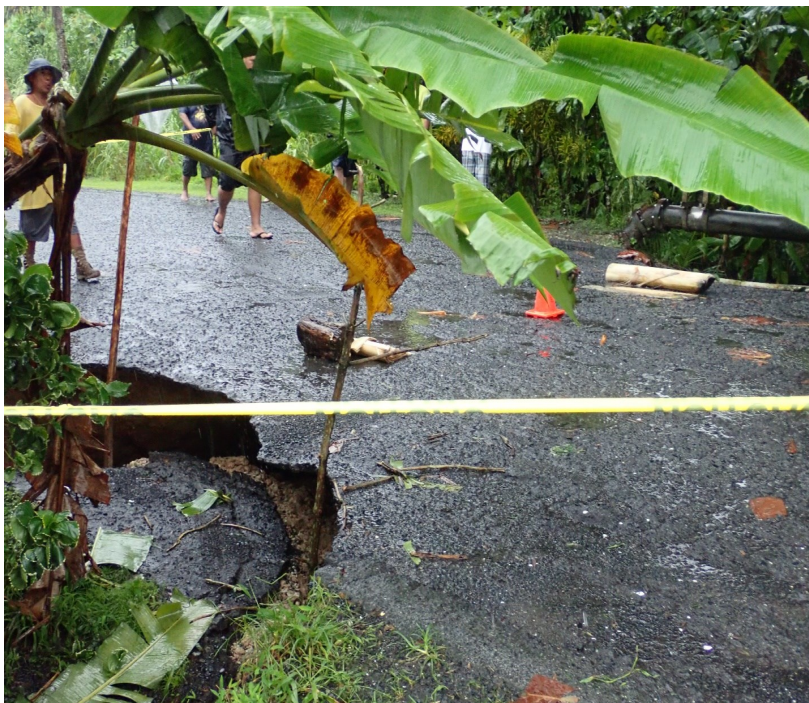
Damage to road in Madolenihmw
