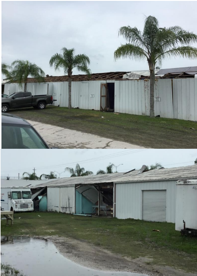
Straight-line wind damage at the Daytona Flea Market (June 6, 2020).
