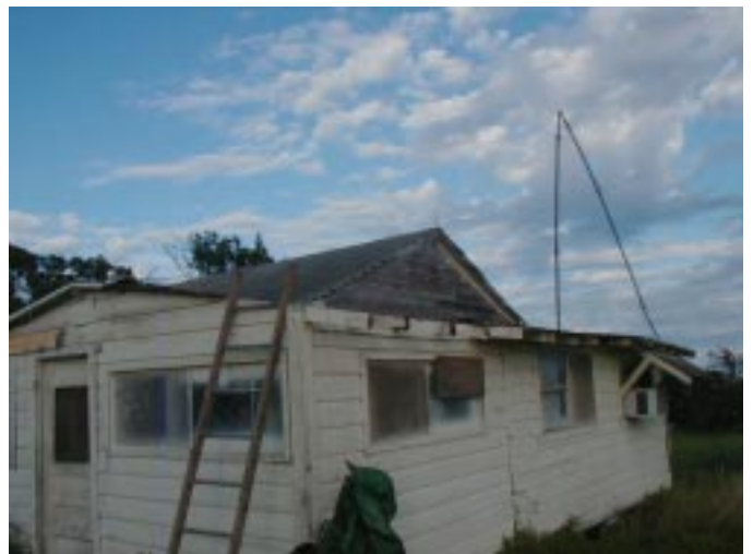
Damage done to home near Millican in southern Brazos County by an F0 tornado on 10/05/03.
