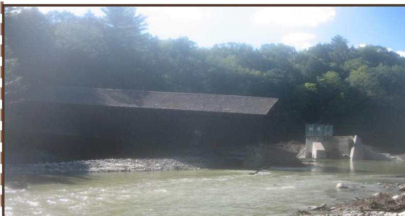
Above: Damage to Eunice Williams Covered Bridge on the Green River at Greenfield, MA.
