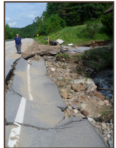
Above: Road damage on Route 9 in NH due to flash flooding on May 29 th .
