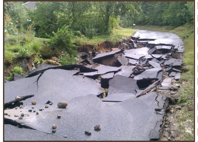
Above: Beebe Road in Monson, MA. had significant damage due to flash flooding on Aug 12th.
