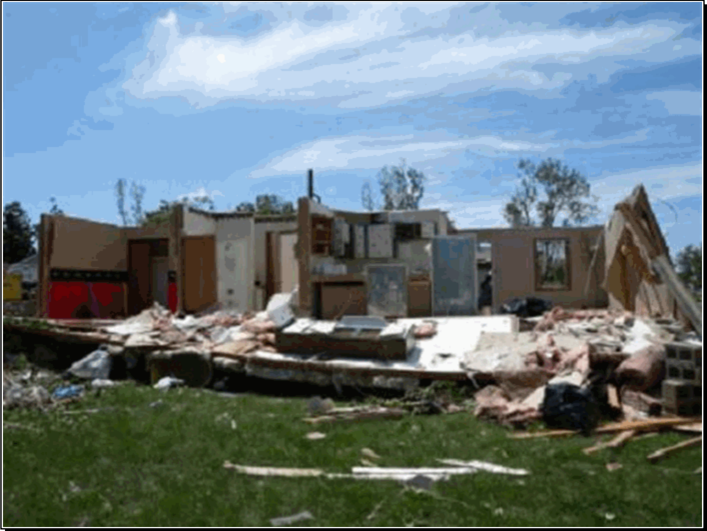
A photo of a destroyed home in Dickinson, North Dakota, on July 9, 2009, the day after an EF3 tornado struck the city. NWS photo.
