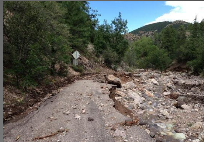
Road Destroyed to Mogollon, NM NWS Damage Survey
